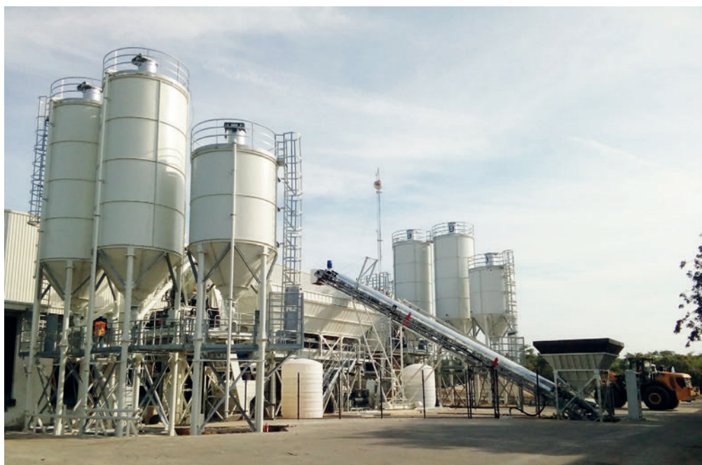
Static plant equipped with two planetary mixers
